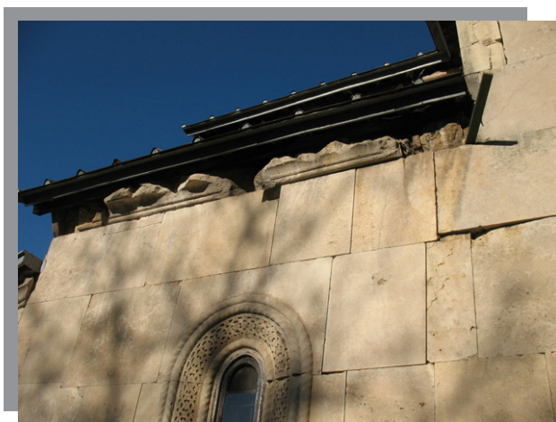
Gelati. St. Giorgi's Church, roof with broken cornices
