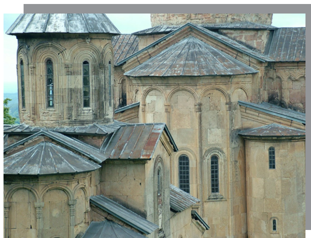
Gelati. Depreciated tin roofs, 2007
